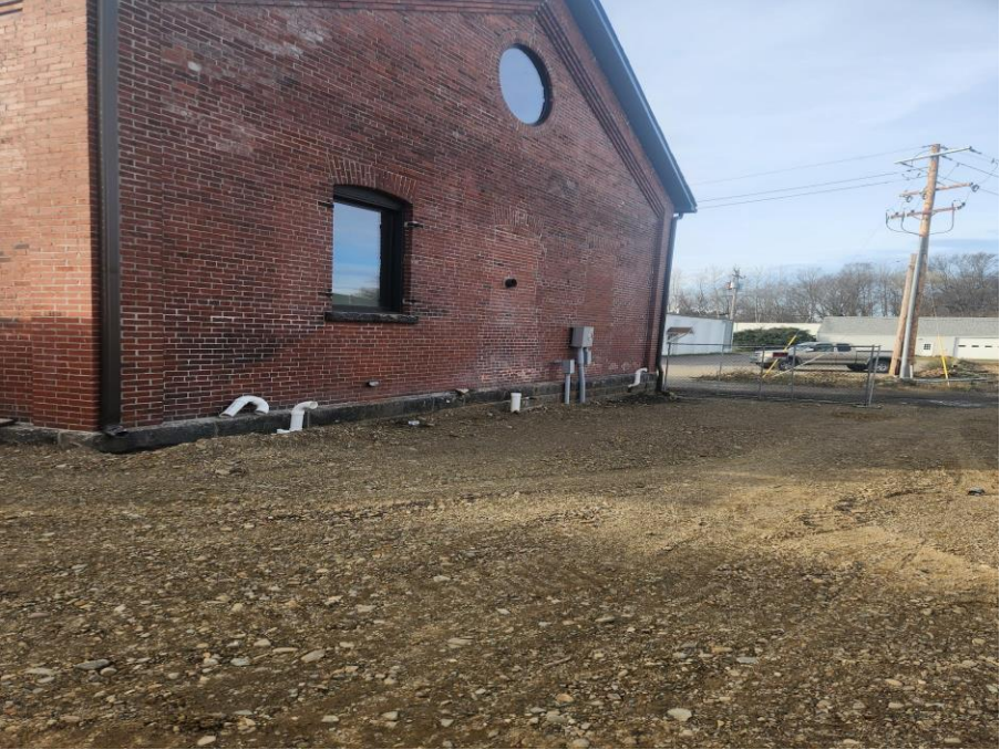
Figure 8. Recommended area for pollinator garden to cover pipes and infrastructure outside building for art studio.
